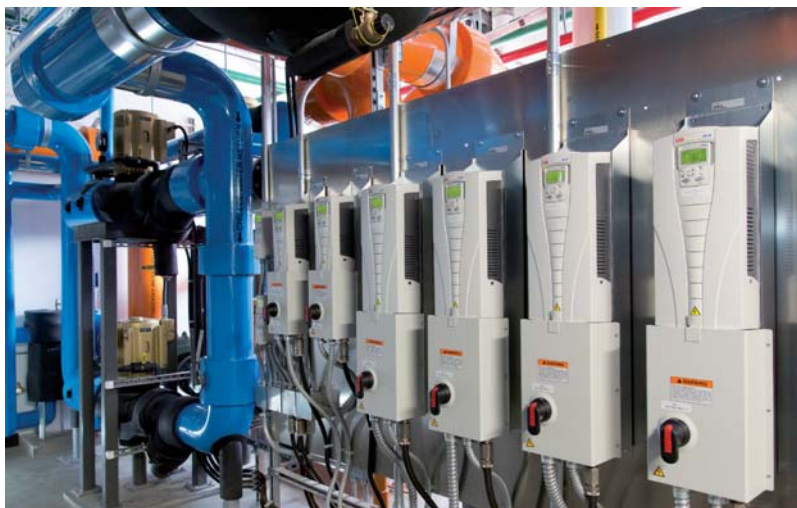
Nearly every device in the highly intelligent and flexible building communicates via BACnet
